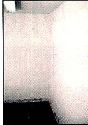
Photo 7. The southeast corner before shielding. The fluorescent light fixture requires bypassing and bonding to the foil.
