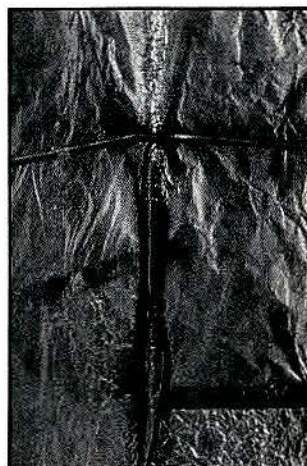
Photo 4. The No. 4 ground wire is bonded mechanically and electrically to the foil at the juncture of both walls and the floor. Foil-backed tape is applied to the entire length of each section's seam.
