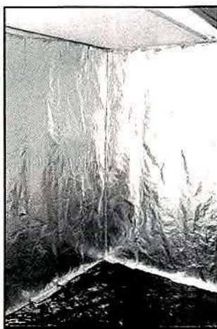
Photo 2. Applying the shielding began by hanging 8-foot lengths of 15-inch aluminum foil directly on the wall. Overlapping pieces are stapled directly to the wall with office paper staples.
