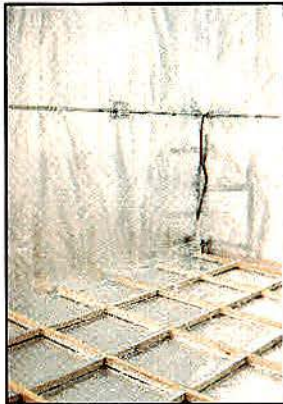
Photo 5. A double-layer of foil on the floor is taped and bonded to the protruding wall foil shown in Photo 2. Liberal use of foil-backed tape virtually hermetically seals the flooring to the walls.
