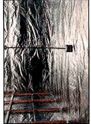
Photo 8. The southeast corner after shielding. The foil, floor support lattice and electrical service boxes are put in place.
