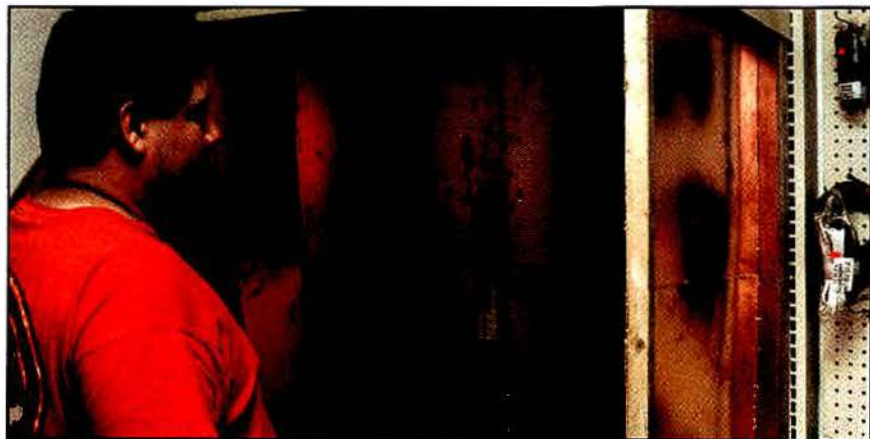
Centrally located, the ac outlet strip is connected to an electromagnetic interference (EMI) filter behind the panel.
