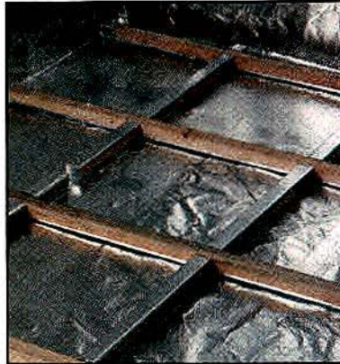
Photo 6. Foil-backed tape covers the bottom of the 2"×2" floor frame of interlocking crosspieces to maintain bonding even if the underlying foil becomes abraded.
